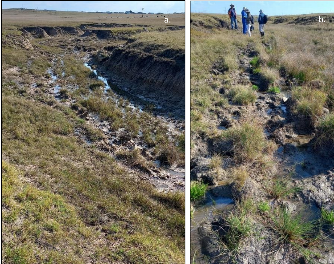
Figure 3-132 The main erosion gully in the wetland (downstream of the headcut shown in the previous photo) with (a.) located shortly downstream with incomplete vegetation cover and (b.) somewhat further downstream where vegetation cover is generally higher and more sediment has accumulated than above but a cattle path has provided a focal point for localized incision and remobilization of some of the deposited sediment
