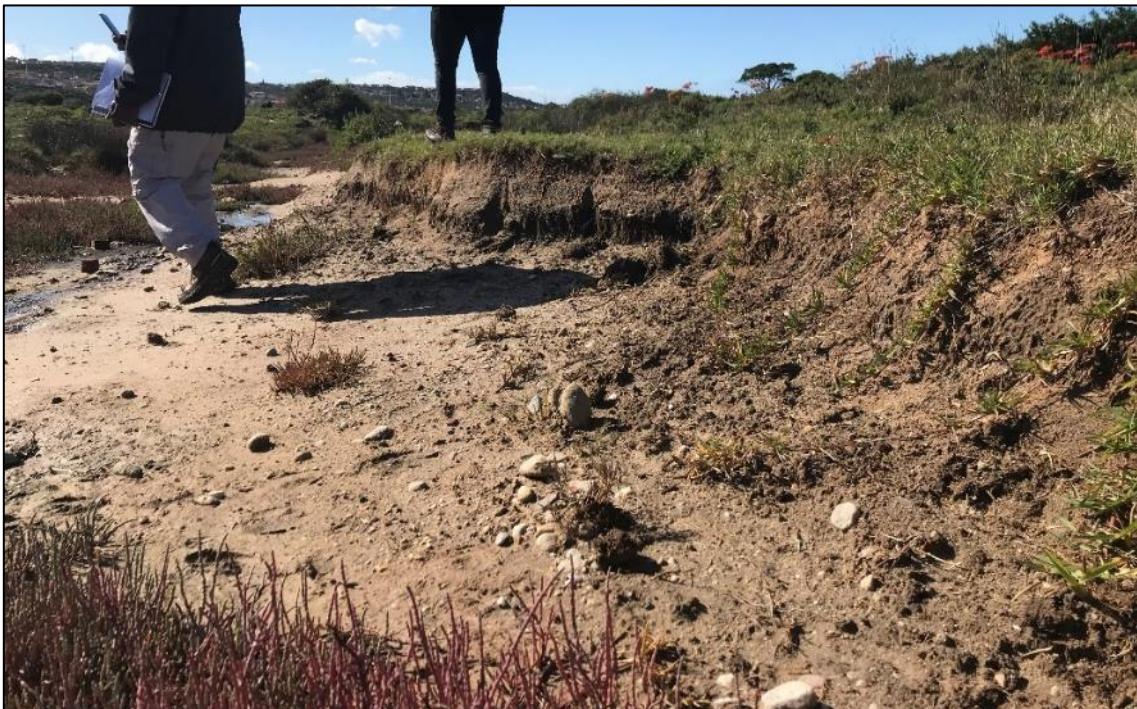
Figure 3-39 A lateral erosion gully that has been created directly downstream of one of the stormwater drains inputting water into the CVB 1 wetland. It appeared to be moderately active, with a stand of Pennisetum clandestinum growing across the active face of the headcut.
