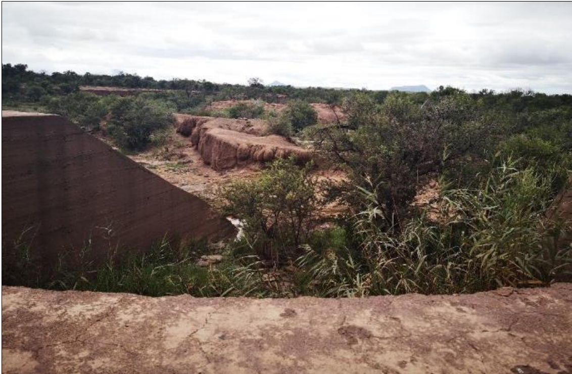
Figure 3-50 View of the erosion gully downstream of a weir
