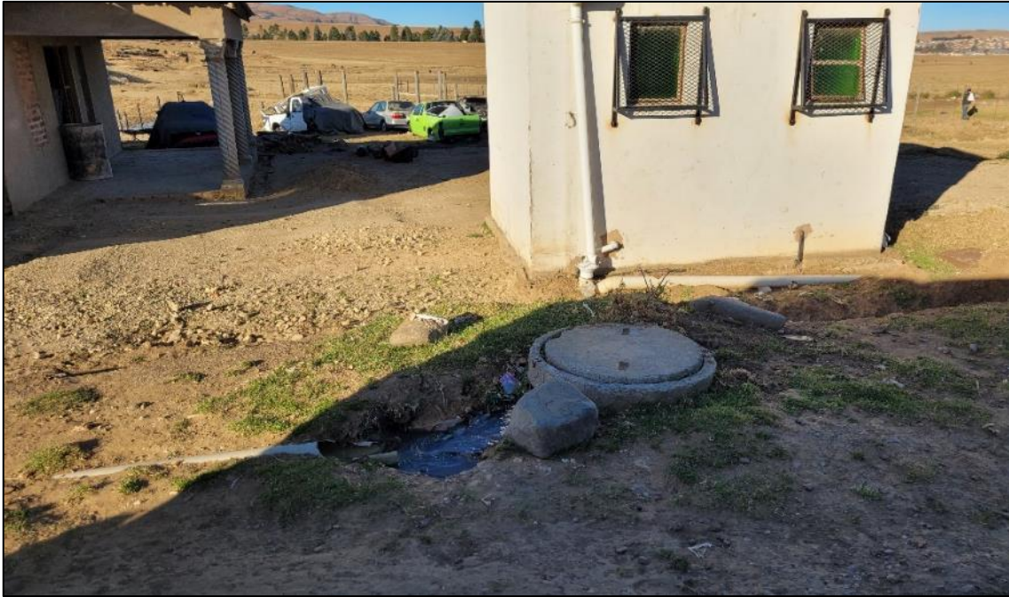
Figure 3-92 Surcharging manhole with the sewage being directed towards the wetland
