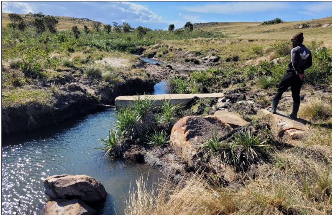
Figure 3-115 Xolobeni wetland: Eroded palmiet wetland upstream of the water supply pipeline crossing point. Portions of the pipeline has been encased in concrete, however the channel has bypassed the concrete and has exposed portions of the pipeline
