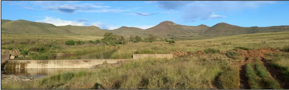
Figure 3-138 An erosion-control concrete weir in a small valley bottom in the Loodsberg foothills, likely constructed several decades ago through Department of Agriculture's soil conservation initiative.
