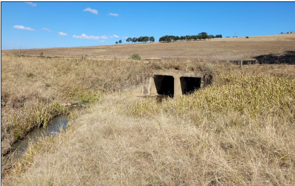
Figure 3-126 View of the road culvert associated with the R61 which has led to the formation of a small headcut erosional feature upstream of the culvert. The headcut has not progressed too far due to the shallow bedrock layer within the system
