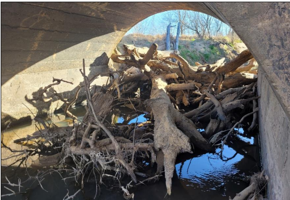
Figure 3-84 Debris below a large road culvert across the incised portion of the floodplain.
